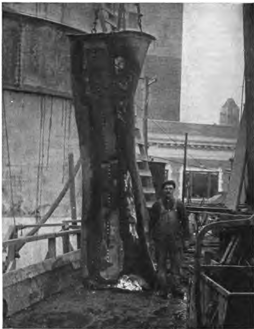
PLATE 232. —Contract 67. Shaft 23. Steel Shafting, Collapsed by External Pressure of Wet Sand while Sinking Caisson.
